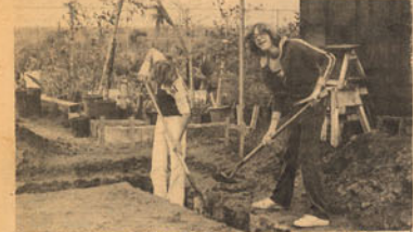
DIGGING THE FOUNDATION for a new storage shed for horticulture are two members of the carpentry class, David Neal, left, and Greg Stachura.
